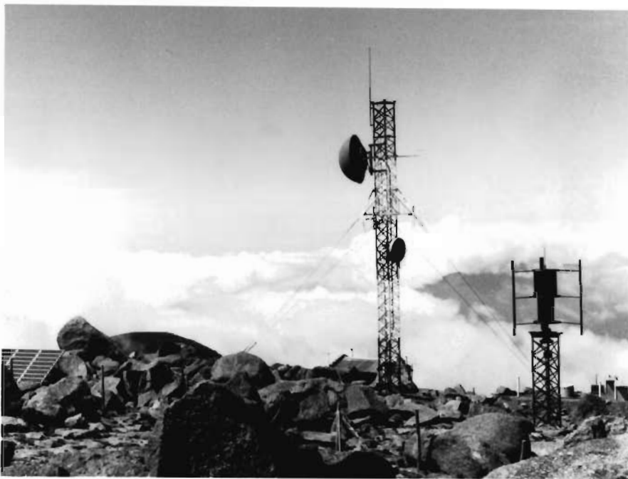
Fig. 1 The CERRO NEGRITO REPEATER located 4500 m above sea level in Argentina has a complete ERIGEN hybrid power system and a datalogger installed.
