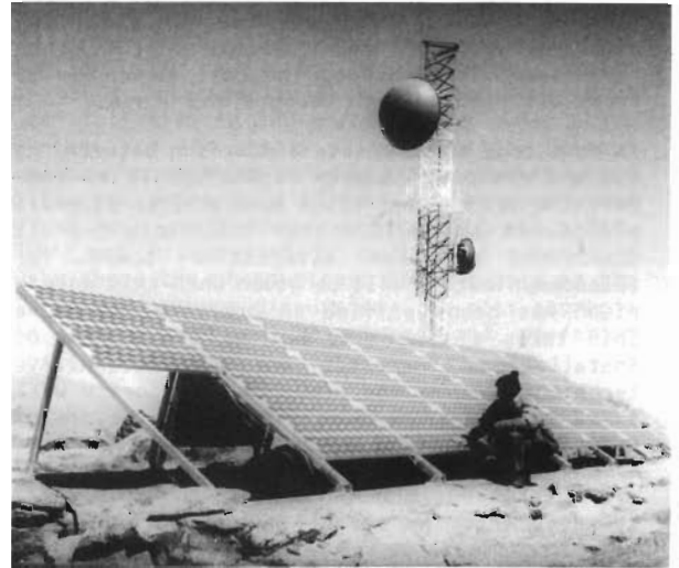
Figure 7. The El Negrito repeater in Tucuman Argentine 4000 m above sea level was built by Ericsson in 1984. All equipment were carried up to the top by men and mules.
