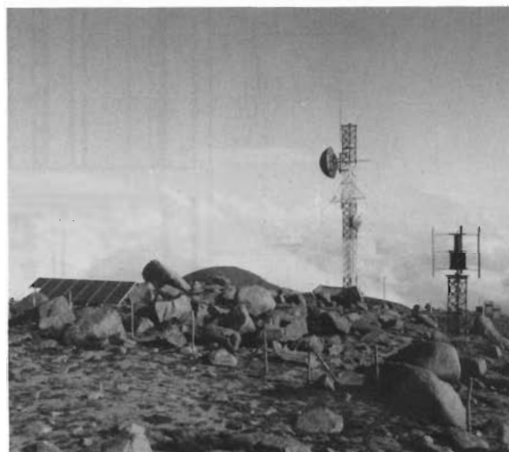
Fig. 1 The CERRO NEGRITO REPEATER, located 4500 m above sea level in Argentina has a complete ERIGEN hybrid power system and a data logger installed.
