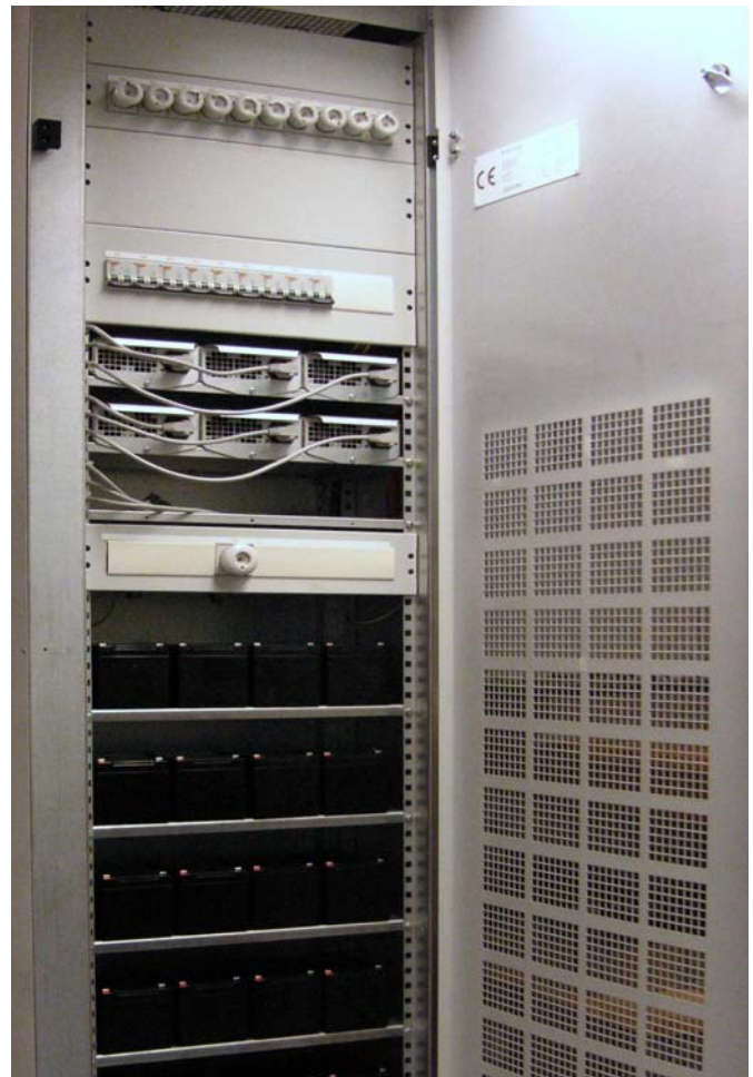
Fig. 5. A 9 kW Netpower HVDC UPS.
